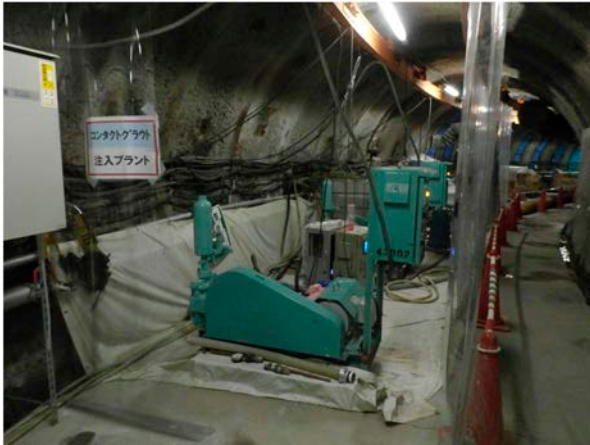
(a) Grout pump
