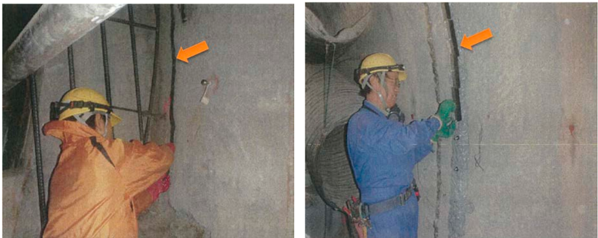
(a) Bentonite strips (b) Grout stopper Photo 98 Setting bentonite strips and grout stopper
