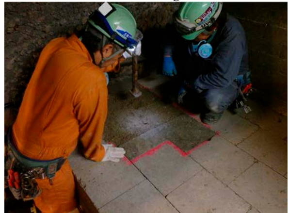
(f) Infilling wireless sensor
